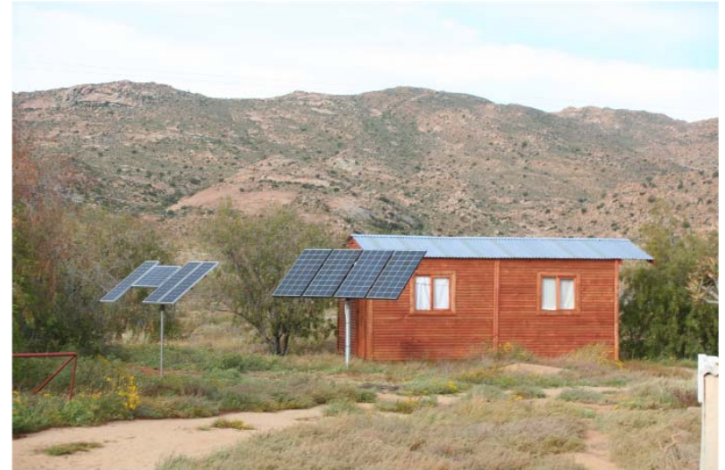
The Wendy house we erected last year where Ivana and Ed live in and the small solar panels erected two years ago, as well as the four small solar pennals we connected to the system now. The big solar panels provide 17 A at 24 V (408W), the small ones 6A (144W).
