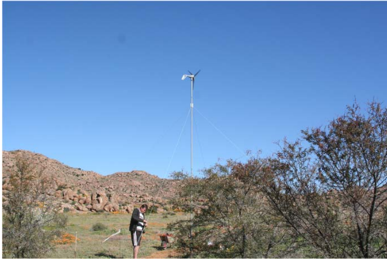
The wind turbine gets erected. It can produce up to 9 A (216W) and this 24h a day!
