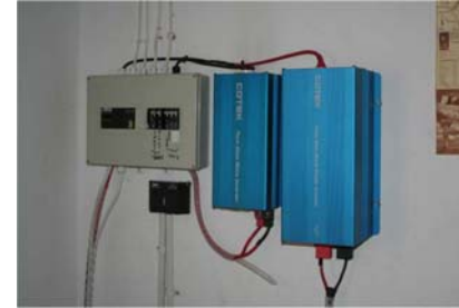
Our fuses and left the old Inverter that can handle 1000W and right the new inverter that can produce even 3000W. Power in the kitchen area comes from the new inverter such that we can use electrical fridges there.
